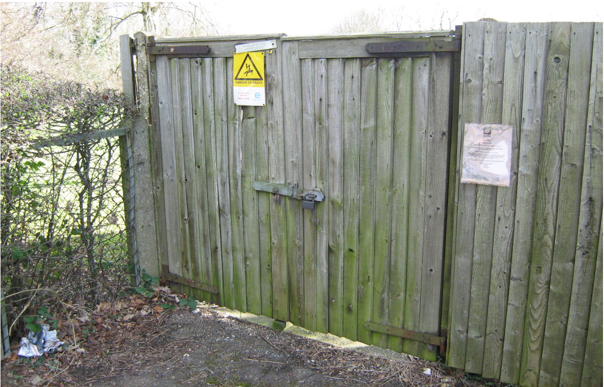
Photo 2 View of the Electricity Sub-Station
